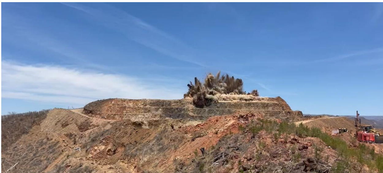
Photo 1 - May 5 th , 2024 – Early blasting of the top of the Nicho Main zone ridge
